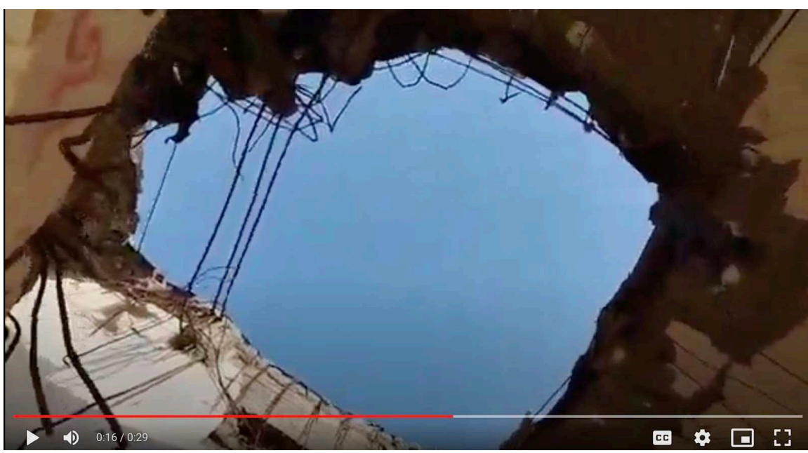
image 28: an installed shot from a video clip shows a hole caused by aerial bombardment of the roof of the school building.
