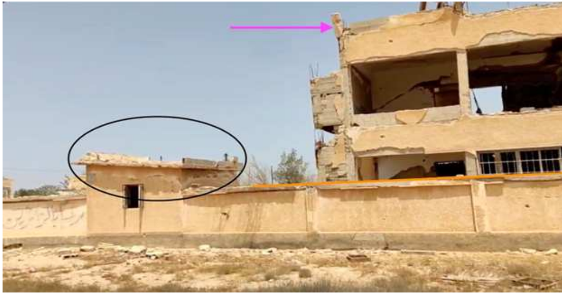
Image 4: Image of the actual dilapidated building, the south wall and a small building on the edge of the school.
